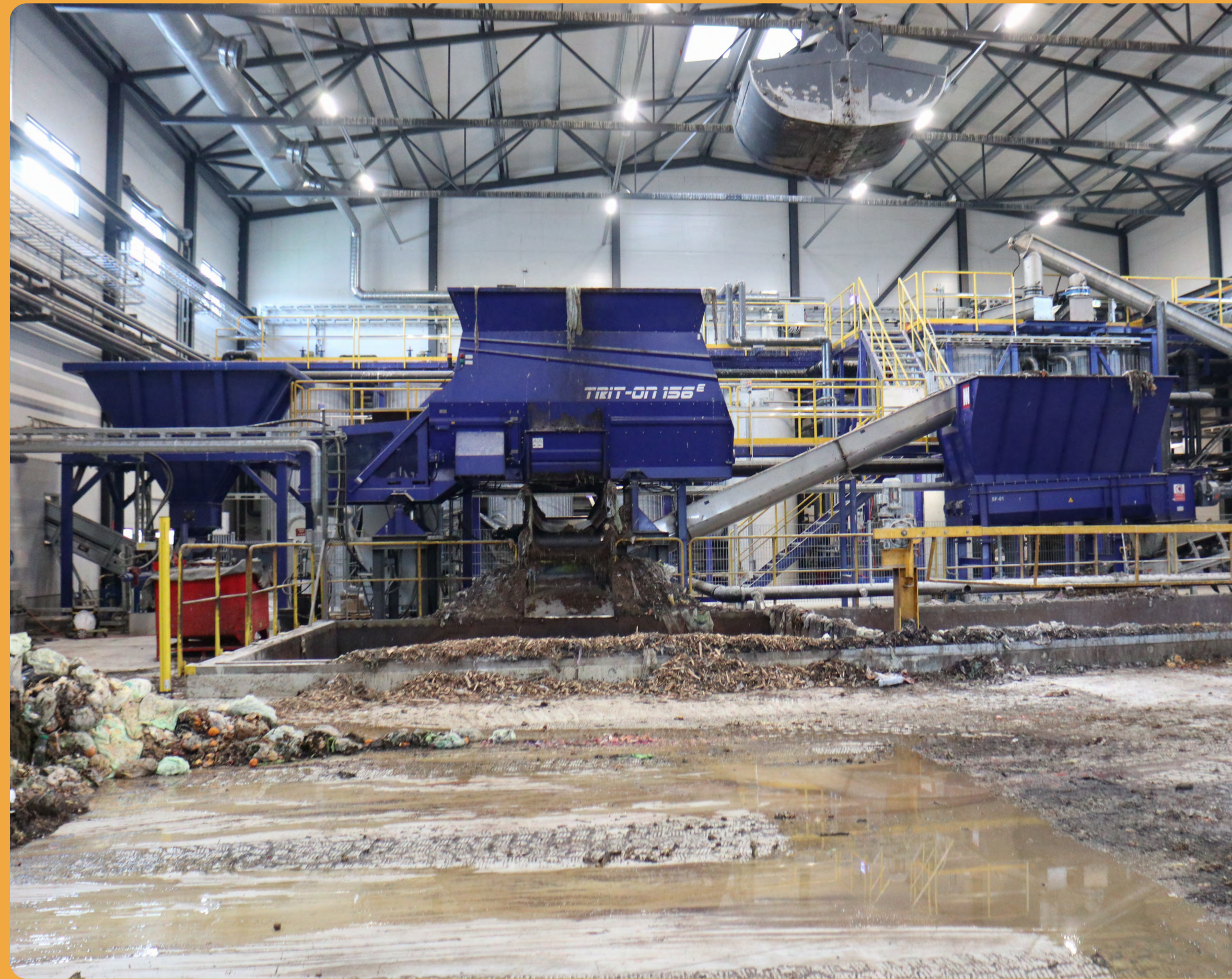
FIGURE 6: DEPACKAGING EQUIPMENT REMOVES ALL PACKAGING FROM FEEDSTOCK
